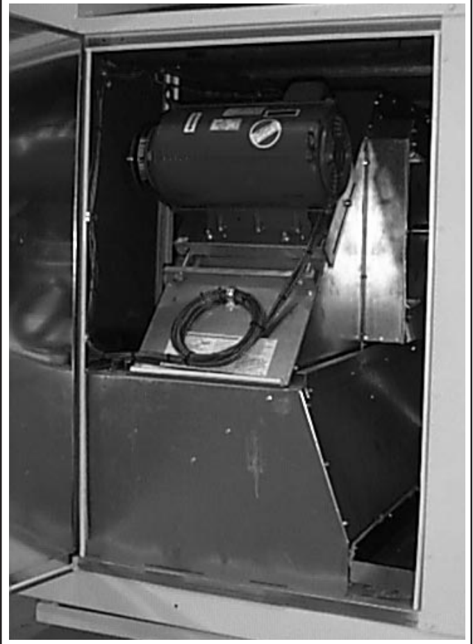
Typical slide-out blower section
