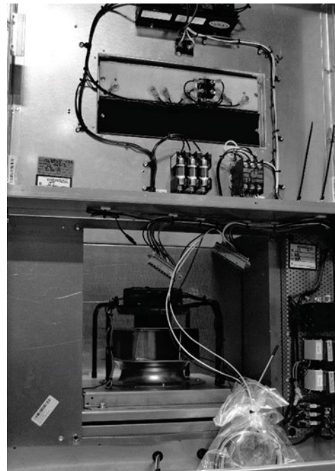
Figure 7: Supply Fan Access after
