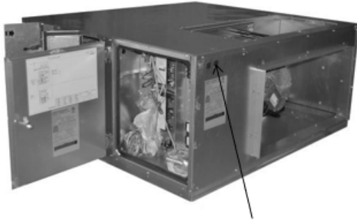
Figure 25: H3 Internal Control Panel Electrical Connections
