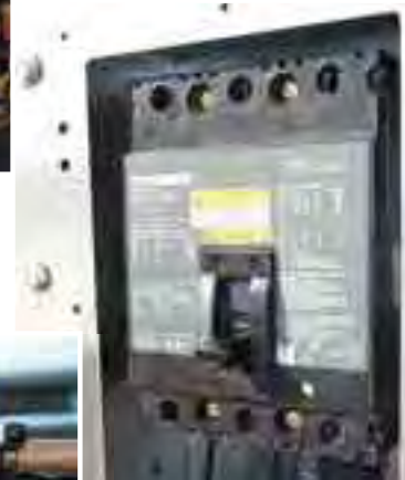
Unit Disconnect Switch
