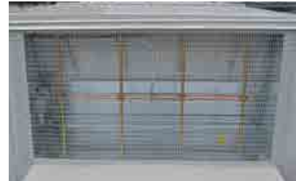
Outside Air Opening with Airflow Measurement System (shown without rain hood)
