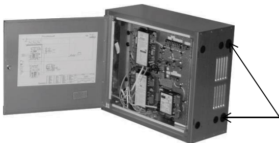
Figure 15 - External control box electrical connections
