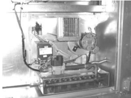
Figure 39- Gas Heat Exchanger
