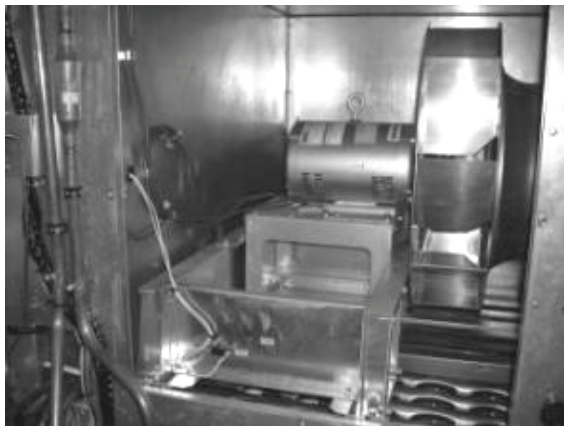
Figure 38 - 11-25 and 30 ton Supply Fan
