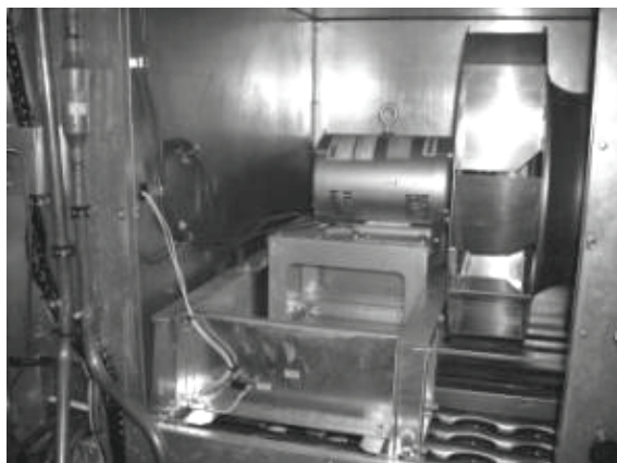
Figure 41 - 9-25 and 30 ton Supply Fan
