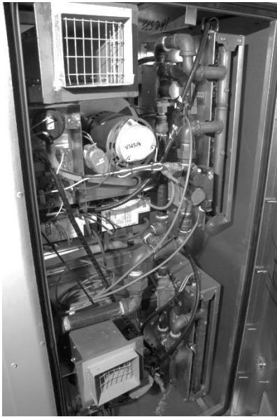
Figure 23 - Gas Heat Exchanger
