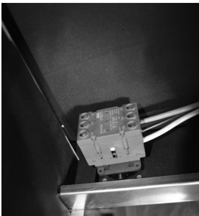
View of a disconnect switch terminal block from the inside of cabinet.
