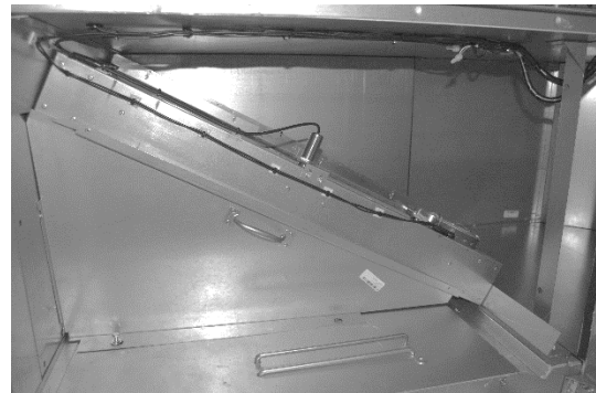
Figure 32 - H3 C Cabinet Outside Air Filter Access
