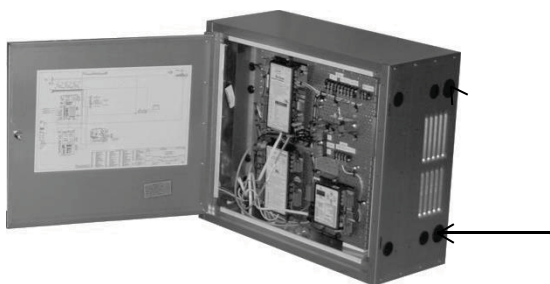
Figure 15 - External control box electrical connections
