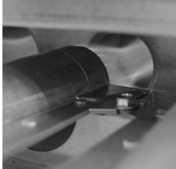
Burner Flame @ Start-up 1.2” w.c. Manifold Pressure Draft Inducer – High Speed
