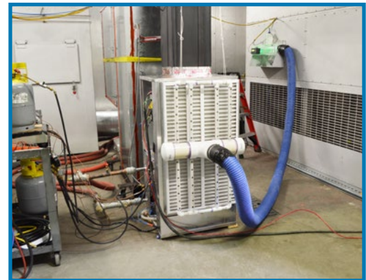
▲ High Tech Water-Source Heat Pump Testing Laboratory
