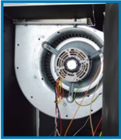
Interior of Supply Fan Section
