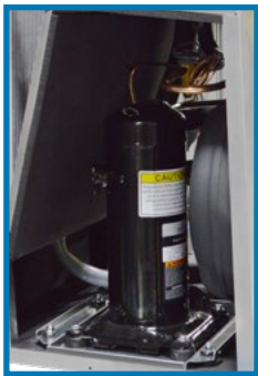
Interior of Compressor and Refrigeration Components Section
