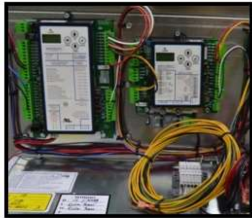
Figure 6 - WattMaster VCC-X Controller and Refrigeration System Control Module
