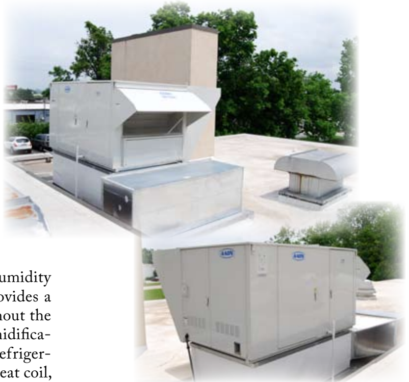
30 Ton Packaged DX AAON Unit with an Economizer and Humidity Control
