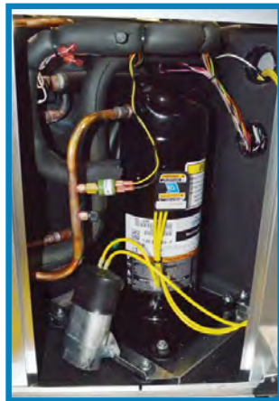
Interior of Compressor and Refrigeration Components Section
