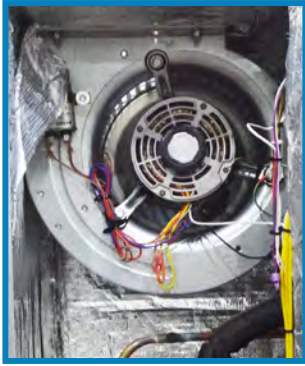
Interior of Supply Fan Section
